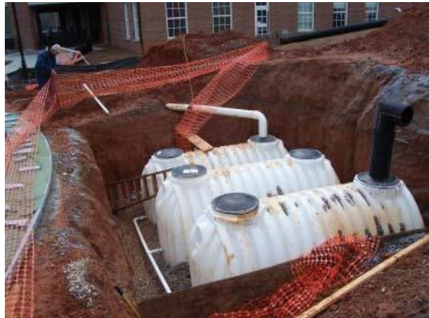
Underground Cistern – Miller Learning Center
